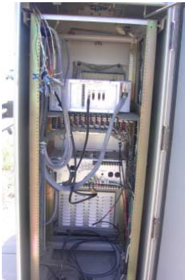
Figure 3.2.3.1. Inside of Type 334c control cabinet containing CAWS traffic monitoring equipment.
