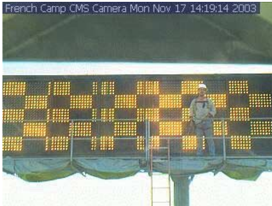
Figure 3.2.4.2. CMS 1 panel replacement, recorded by our CMS verification camera on Nov. 17, 2003.
