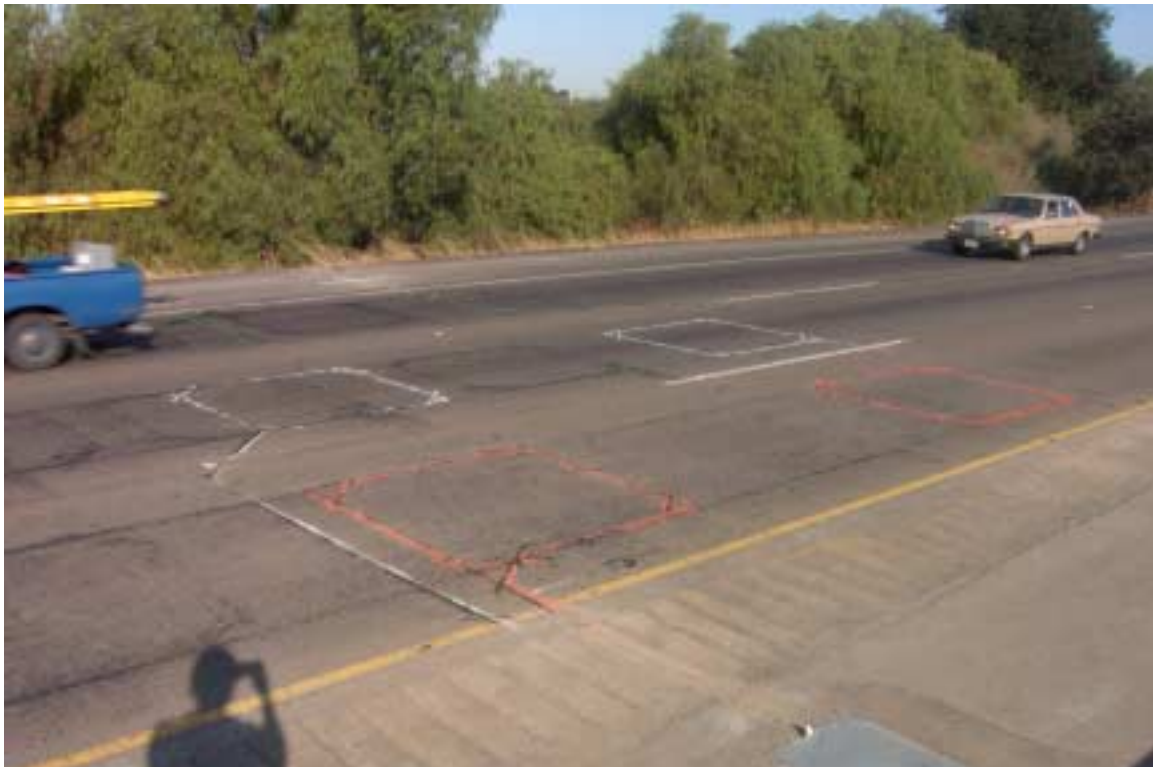
Figure 3.2.3.2. Duplex inductive loops installed in each lane for speed measurement at each traffic monitoring station.
