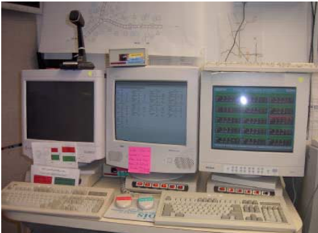
Figure 3.2.1.1. CAWS computers. From left to right: Signview/CAWS, Qualimetrics-Caltrans Meteorological System (QCMS), Traffic Monitoring System (TMS).
