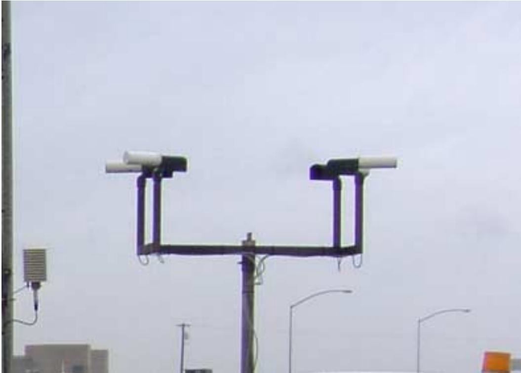
Figure 3.2.5.3. Qualimetrics Model Z004510 forward scatter visibility sensor (center) and Model 5140 temperature/humidity probe (left), installed at each remote weather station in the CAWS.
