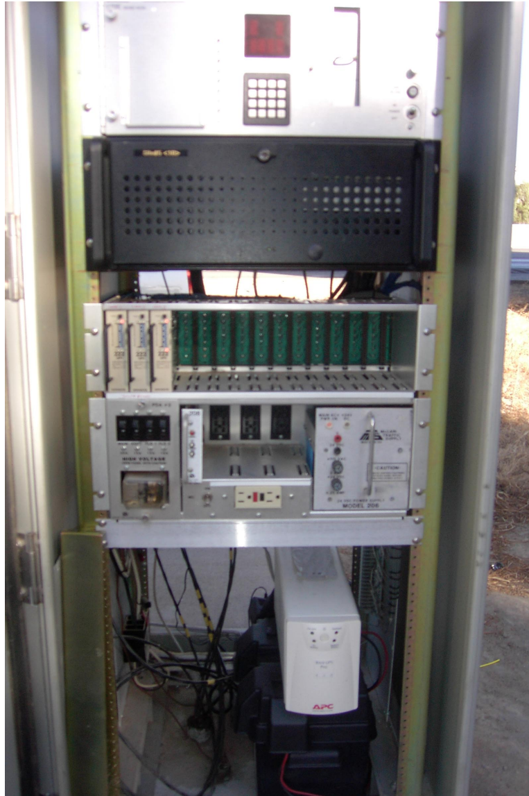
Figure 5.2.3.4. Typical installation of field data acquisition computer and UPS in Type 334-C cabinet.
