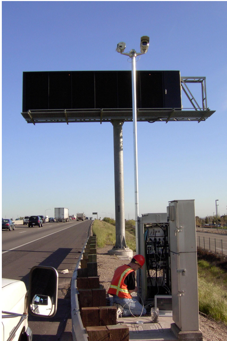
Figure 5.2.3.6. CMS and traffic monitoring cameras at CAWS CMS No. 1.
